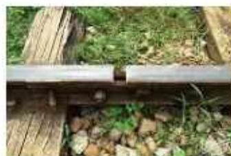
Fig 9.13 Gaps between Rail Tracks
