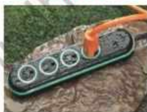
Fig: 15.24 Electrical extension placed damped environment
