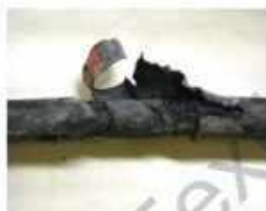
Fig: 15.23 Over heating of a cable
