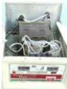
Fig: 16.20 Transformer in stabilizer
