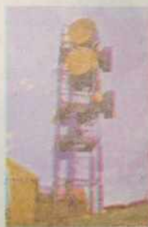
Figure 15.30: Microwaves relay station
